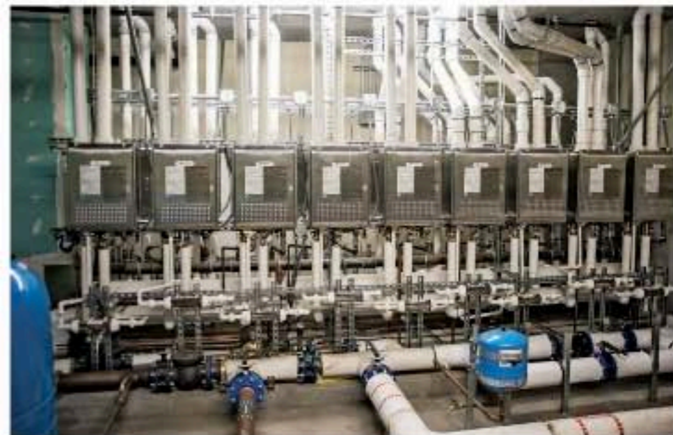
Kevin Hunt, ACCO Engineered Systems' lead plumbing engineer, designed and installed the system at AVA 55 Ninth. He created a unique rack in the middle of the mechanical room where the Noritz NCC-1991-DVC water heaters are mounted back-to-back with the PVC piping run in the middle.
